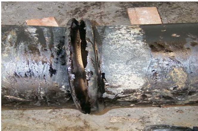
Fig. 1 – Failure mode of the pipeline wall
